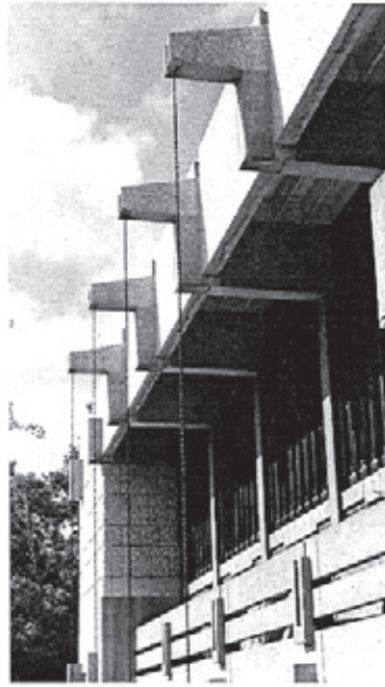
Vertical chains direct rain water to the ground.
